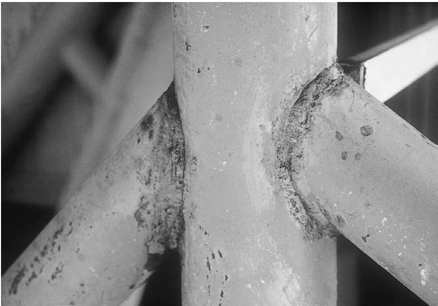
Figure 13.1 Corrosion at weld, largely due to roughness of the weld profile.
