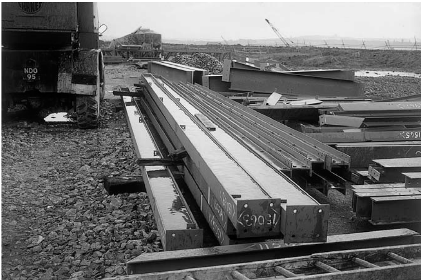
Figure 8.2 Incorrect storage gives an aggressive start to the life of primed steelwork.
