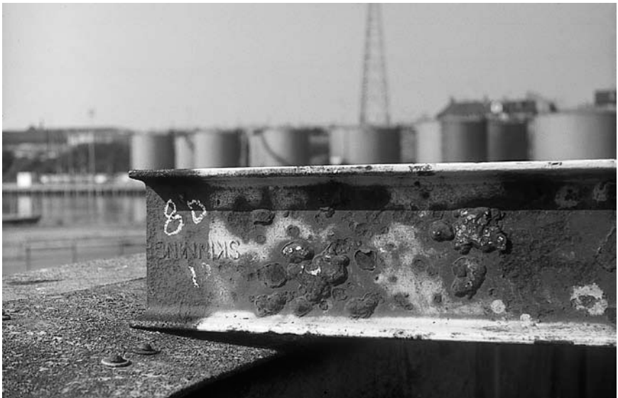
Figure 13.8 Blister from corrosion of the substrate.
