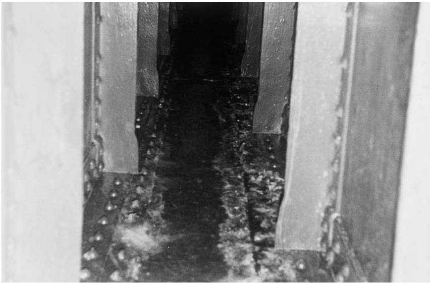
Figure 11.5 Corroded special areas.
