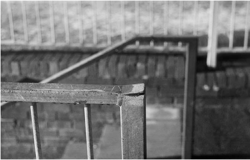
Figure 7.5 Failure at weld on galvanised railings.
