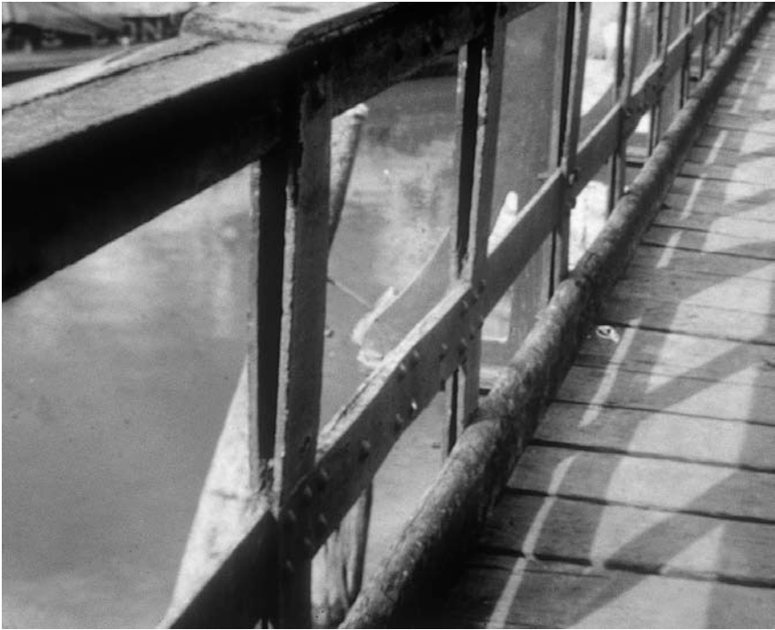
Figure 10.4 The effect of crevice corrosion.
