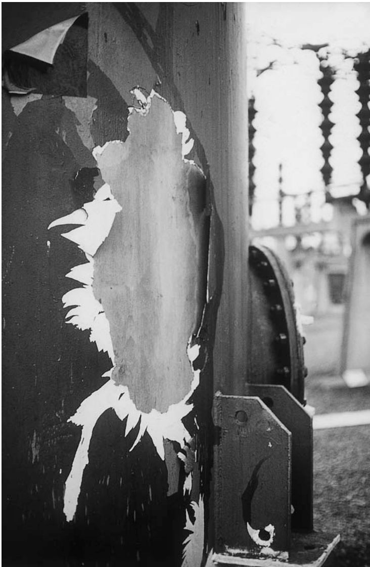
Figure 3.1 Flaking of paint from surface contaminated with grease.
