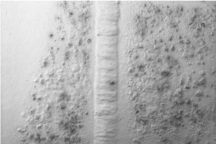
Figure 13.10 Corrosion blistering at overlap between old and new paint at a spot-blasted area.
