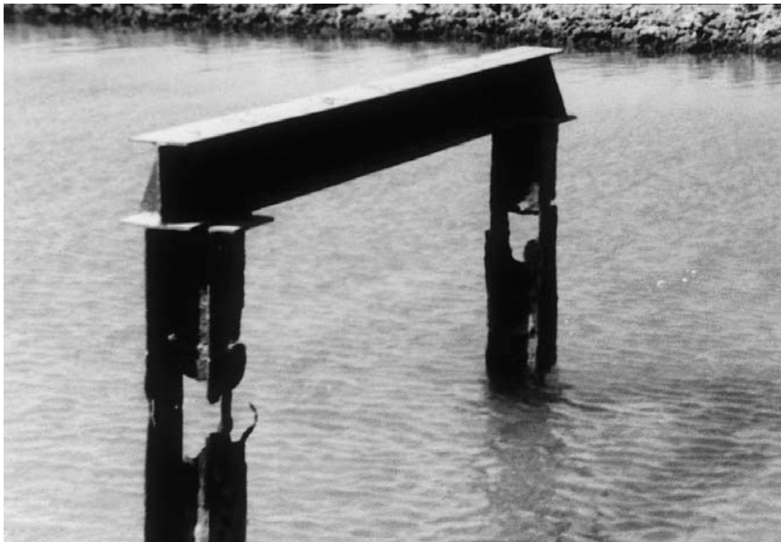
Figure 2.4 Corrosion in splash zone.
