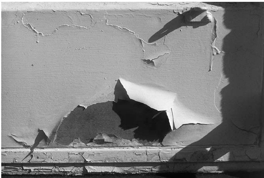
Figure 13.5 Loss of adhesion due to painting over zinc corrosion products.
