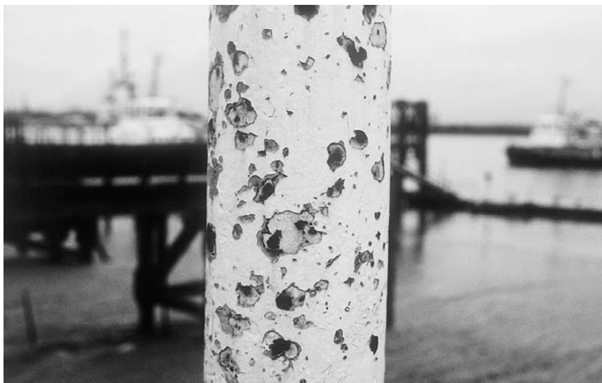
Figure 3.3 Blistering of paint resulting from the presence of soluble iron salts under the coating.
